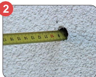
2 Insert tube, or measure depth of hole from finished render back to the original substrate, adding an allowance of 3-4mm to allow the neoprene washer to compress and provide a seal when installed.
