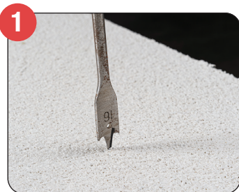
1 Drill a 16 -18mm hole through the render and insulation until the original substrate is reached.
