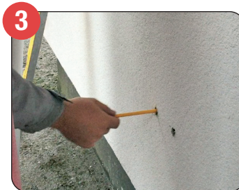
3 Insert tube, or measure depth of hole from finished render back to the original substrate. Allow for the depth of the WL bracket and an allowance of 4mm for the neoprene washer to compress and provide a seal when installed.
