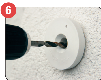
6 Drill through tube into substrate to the appropriate depth for fixing (you may require the use of the washer supplied, dependant on fixing used).
