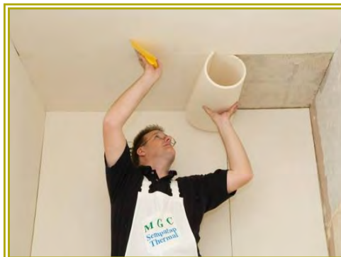
Sempatamp (flexible thermal lining) being applied to walls and ceiling. Source: Mould Growth Consultants
