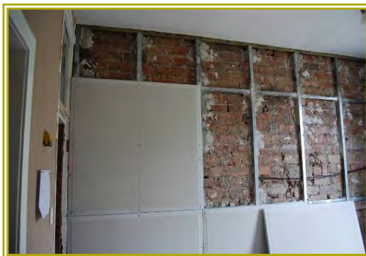
Metal frame fitted onto wall with insulating plasterboard. Source: Historic Scotland presentation
