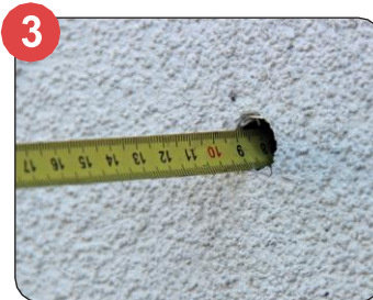
3 Insert tube, or measure depth of hole from finished render back to the original substrate, adding an allowance of 3-4mm to allow the neoprene washer to compress and provide a seal when installed.
