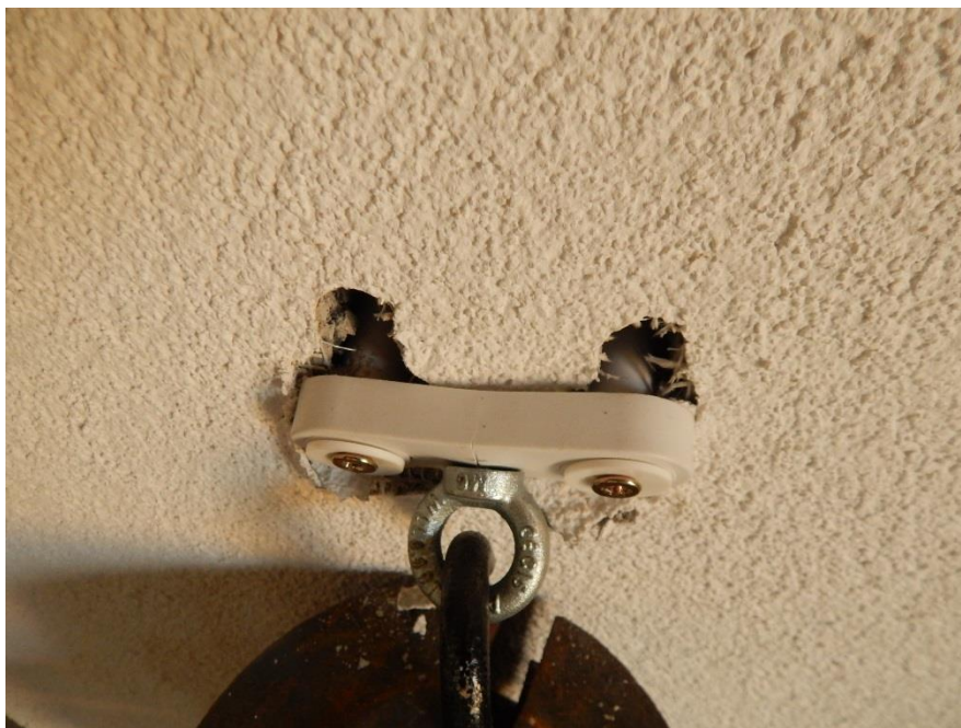
Figure 3 – Fixing failed at this point, (see table 2) notice the cracking of the bracket.
