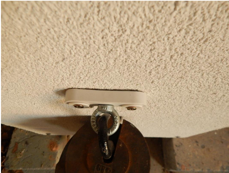
Figure 1 – Fixing starting to come away from surface.
